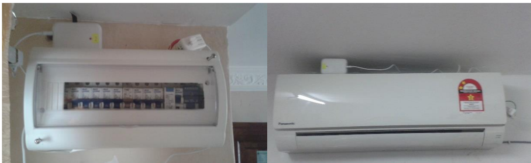
Figure 1. Installation of power monitoring device at a miniature circuit breaker (left) and an air conditioner (right)
