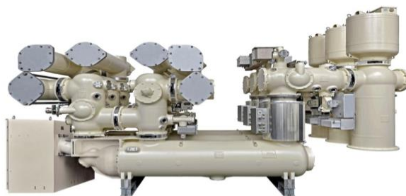
Figure 9. SIEMENS HIS SF 6 switchgear
