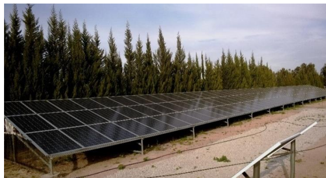
Figure 2. Installed solar panels
