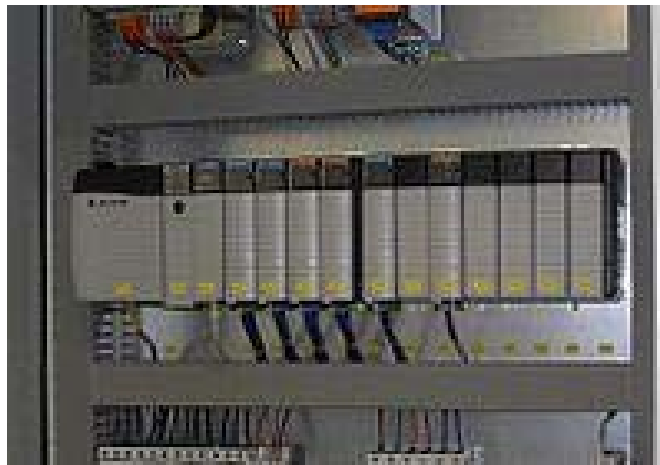
Figure 3. Allen- Bradley Programmable Logic controller
