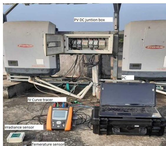
Figure 4. Experimental framework of grid connected PV solar using I-V curve tracer
