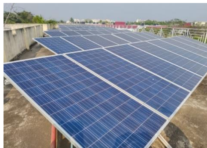
Figure 2. 50.4 kWp grid tied rooftop solar plant
