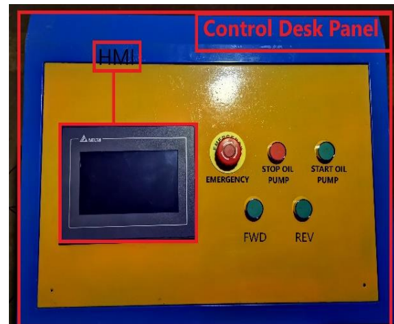
Figure 9. Control desk panel
