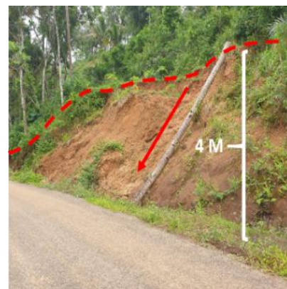
Figure 5. Small landslides on the side of the road in Bubakan Village, Tulakan Sub-District
