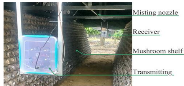
Figure 9. System installation in mushroom cultivation growing house
