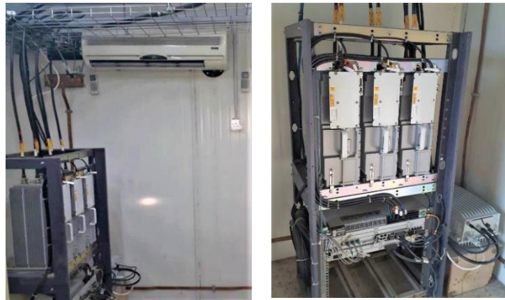
Figure 7. The inside of the BTS shelter room and its component
