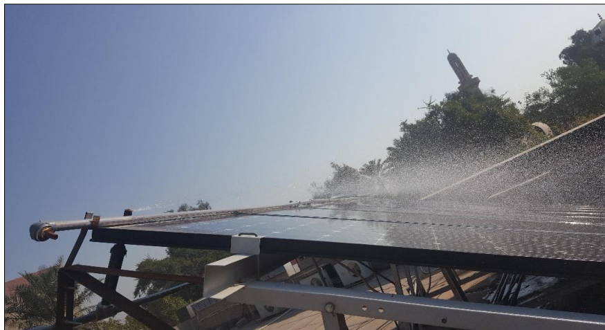
Figure 4. Working automatic-sprayer cleaning system
