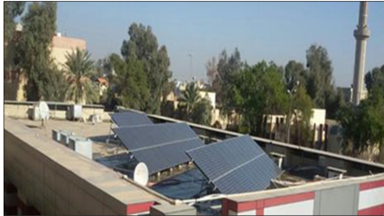
Figure 1. The grid-tied solar PV system of 15 kW
