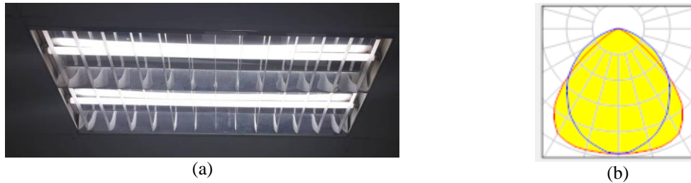
Figure 3. (a) Lighting system fitted a t the ceiling (b) Light distribution curve for selected luminaire
